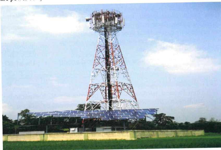
Hybrid power supply to telecom towers
